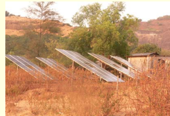
5 kWp Village power, Maharashtra
